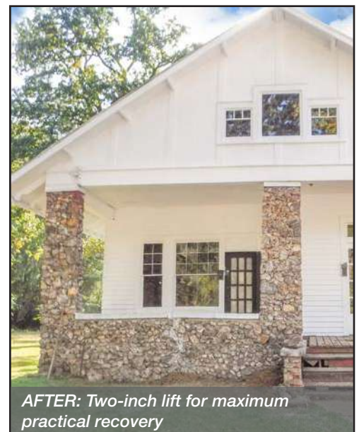
BEFORE: Porch and column settlement
